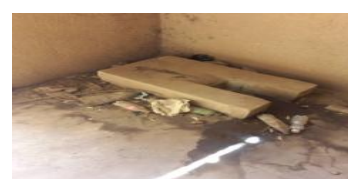
Picture 4: State of the Magnambougou projet A toilet
